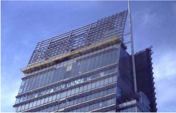
Fig. 6. Bamboo scaffolding at the top of a new high-rise building in Hong Kong [photo: Andy van den Dobbelsteen].
